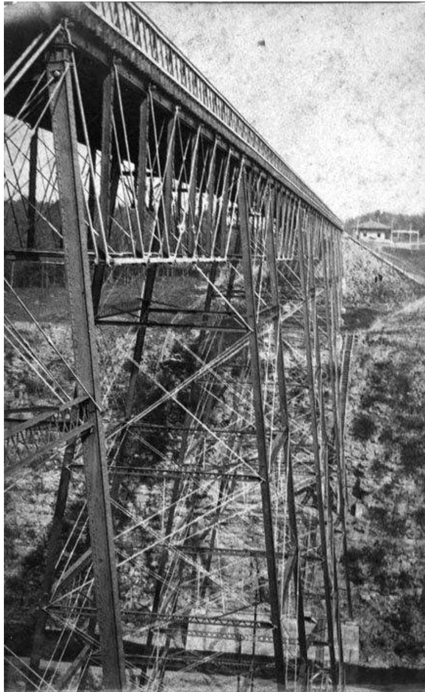
Figure 12. Photograph of Portage Viaduct looking east showing 118' long Span 11 Pratt deck truss. Date unknown (ca.1875-1903). Source: Norfolk Southern Railway.
