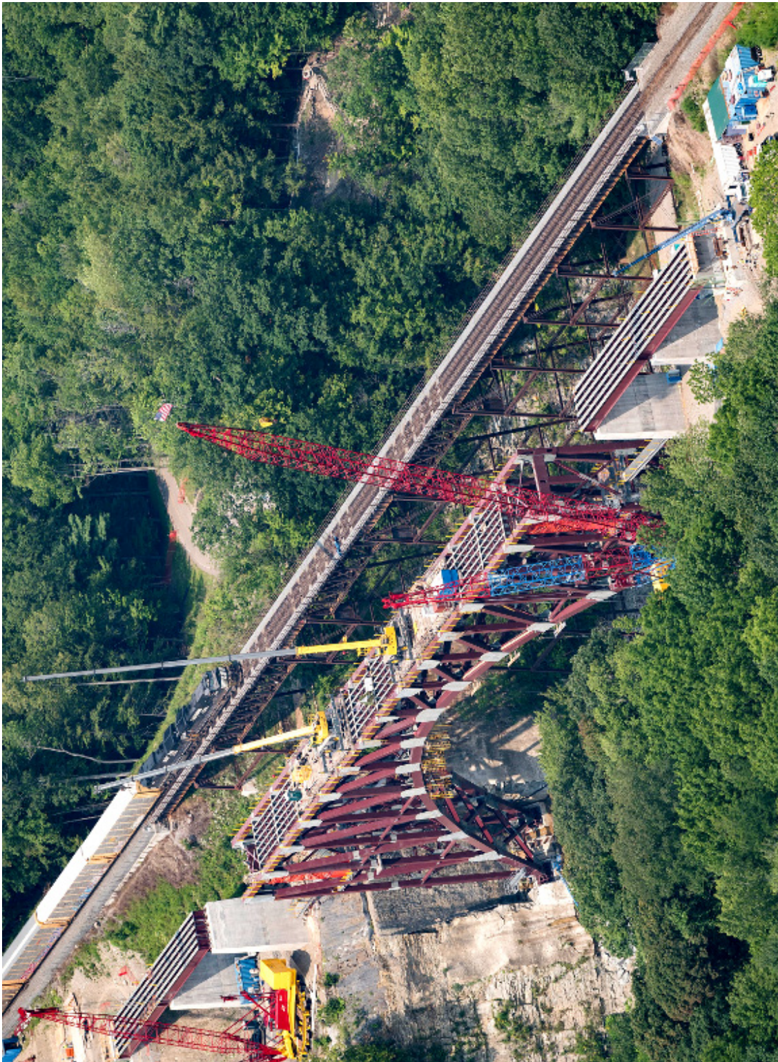
Figure 34. Eastbound Norfolk Southern freight train crossing 1875 Portage Viaduct during construction of the adjacent replacement arch bridge. Aerial photograph by Daniel Spitzer, MD, August 9, 2017.
