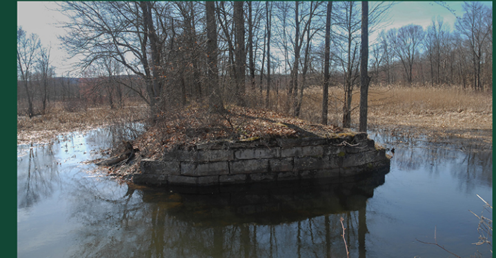
▲ ORIGINAL RAILBED An 1889 Maybrook Line bridge abutment stands surrounded by Black Creek floodwaters. Abandoned 1889 railbed cuts and fills are still visible along the rail trail between South Chodikee Lake Road and Centerville. The Woods Walk Trail, built on a portion of the 1889 railbed, begins at the nearby steps and rejoins the rail trail a quarter mile to the east. Source: Milestone Heritage Consulting.
