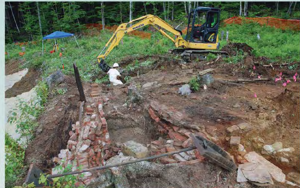
Archaeologists digging with hand tools and a small backhoe documented the workings of the copperas factories as part of the site cleanup. The brick pit in foreground is part of a copperas cooling and settling vessel found at the lower factory in 2009. Source: U.S. Environmental Protection Agency.
