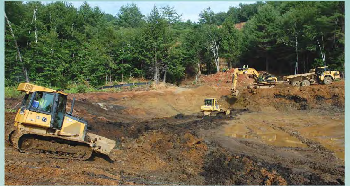
Below: Mine Road looking west in 2009. The EPA removed lead-contaminated soil, reconstructed the road and Copperas Brook channel, and marked the copperas factory sites for public viewing, with a layer of rounded stone matching the original ground contours. Source: U.S. Environmental Protection Agency.
