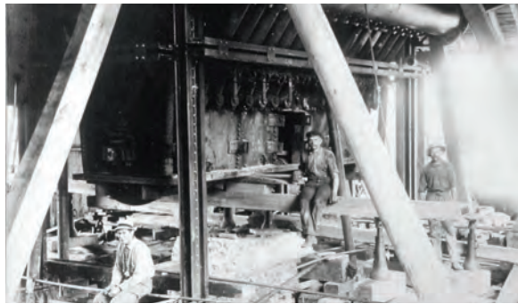
Vermont Copper Corporation blast furnace under construction, about 1908. The main air blast pipe and row of individual blast nozzles are visible above the detachable hearth. Source: Strafford Historical Society.
