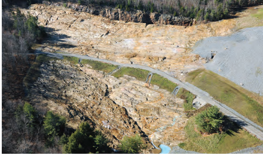
Once TP-3 was scraped clean, Copperas Road was reconstructed across it, and rock-lined drainage culverts were installed. Historic diagonal bedrock trench made to direct weak liquid copperas to the factories is clearly visible below the road. Waste removal resulted in over 95 percent reduction in copper discharge from the hillside. Source: U.S. Environmental Protection Agency.
