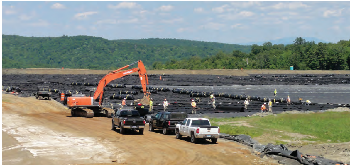
Once mine waste was consolidated on the tailings pile area, it was graded to shed water, and covered with an impermeable plastic barrier, which is being unrolled and sealed in this view across the top of the capped waste. The plastic barrier was then buried under two feet of soil. Source: U.S. Environmental Protection Agency.
