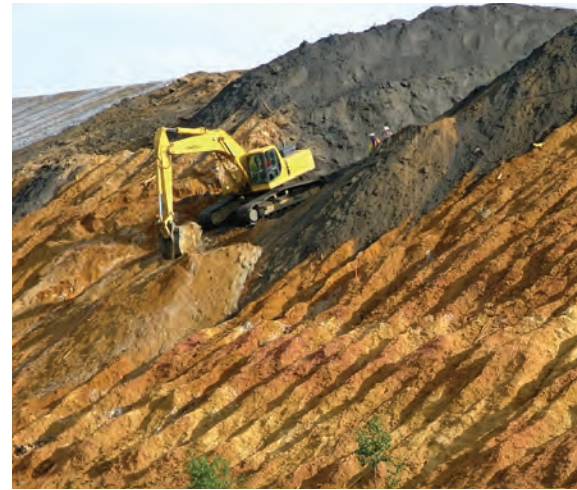
To prepare TP-1 for the waste repository, its steep, eroded sides were regraded for stability. Excavation revealed the unoxidized black pyrrhotite (iron sulfide) under the weathered outer orange layer of tailings. Source: U.S. Environmental Protection Agency.
