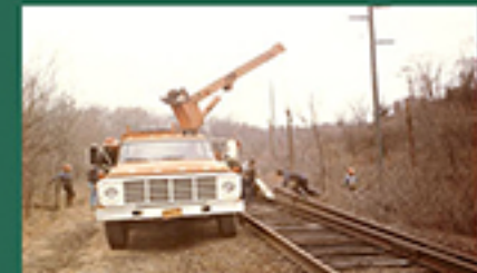
▶ END OF THE LINE Sculpture workers tore up the Maybrook Line tracks in Lloyd in 1982, the year after rail service ended here. The Hudson Valley Rail Trail Association opened the first short section of the Hudson Valley Rail Trail on the Maybrook Line right-of-way in 1997. The trail has expanded east and west and become a segment of the 750-mile-long Empire State Trail in 2020. Source: Austin McInerney photo, Vision News Service collection.
